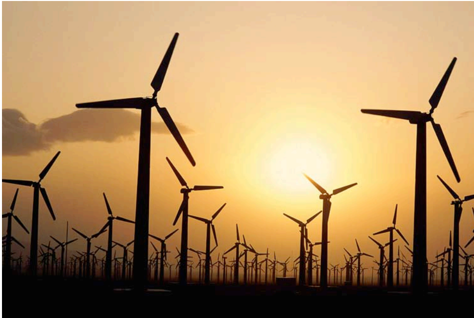
Photo 24. Fiber optics is used to transfer data at this wind-powered electric generating site because of low weight and noise-free transmission.
