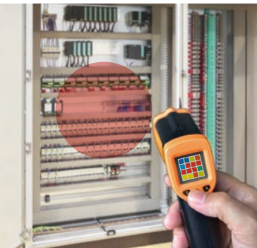
Transformers & distribution boards
